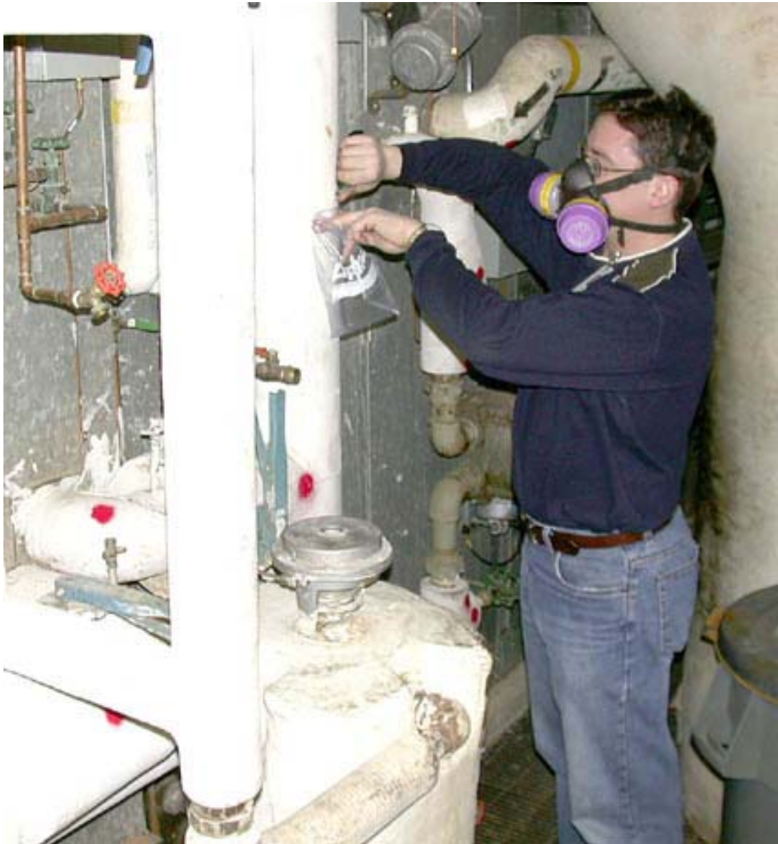
Consultant Clint Berschiminsky checks for asbestos in pipe insulation in a mechanical room in the U of S Health Sciences Building recently. Berschiminsky is conducting an inspection of all campus buildings.
