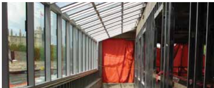
Window wells in the Place Riel addition will provide natural light to all floors.
